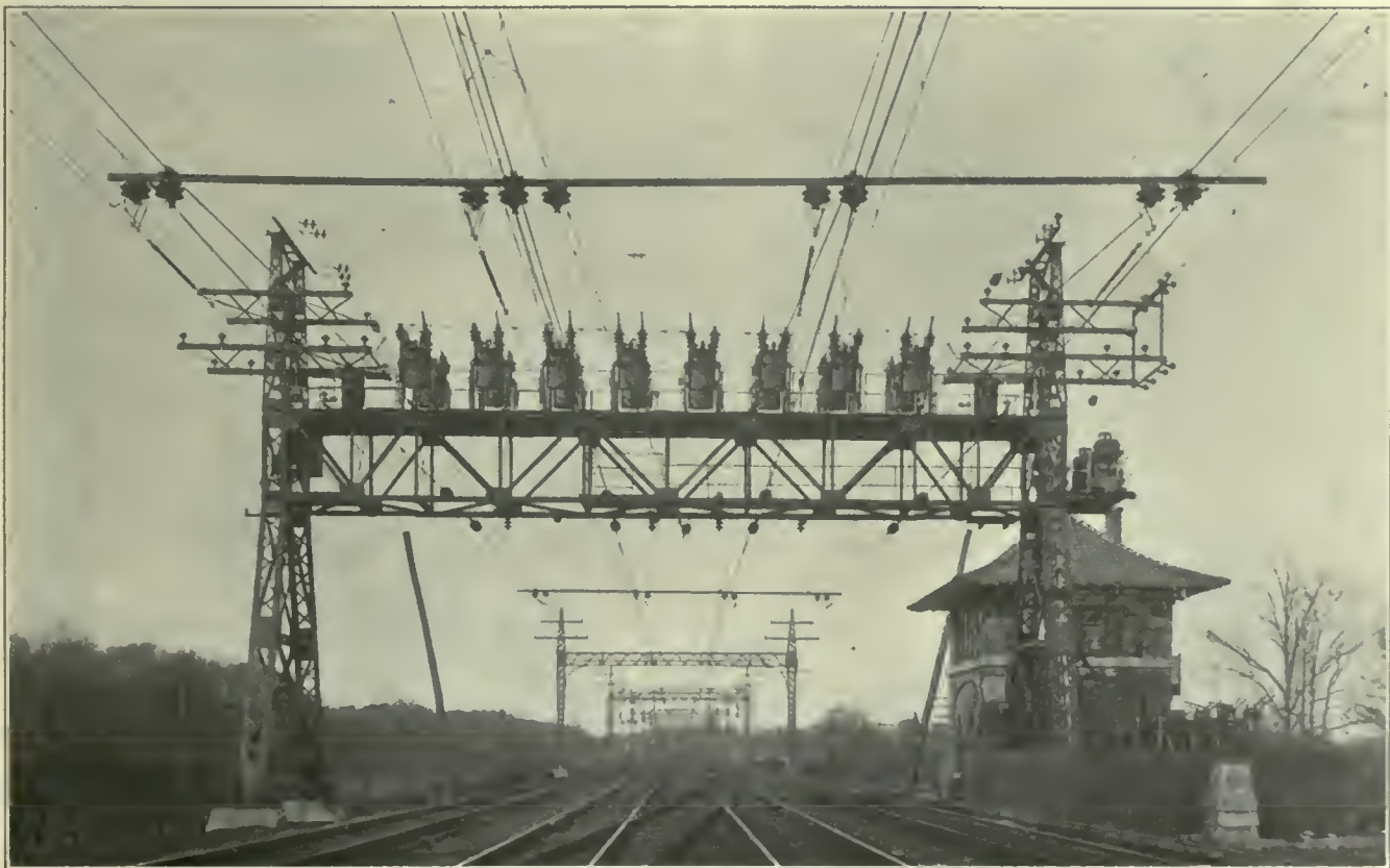
FIG. 520. OVERHEAD CONTACT SYSTEMS. Anchor Bridge and Electric Switching Station, New York, New Haven & Hartford Railroad.
